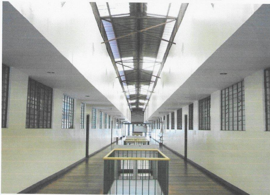
VENTILATION AT CHARLIE BUILDING
